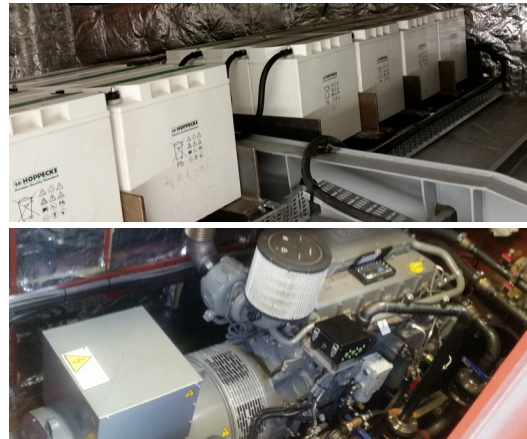
DC supply from a battery pack or generator AC supply, or both.
